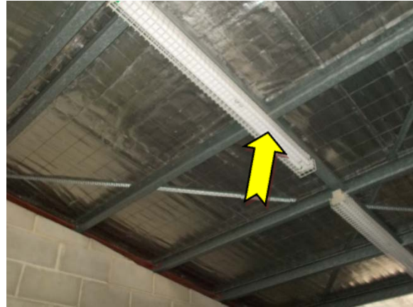
Photo 2. Interior, fluorescent double tubed light fitting – suspected non PCB-containing capacitor.
