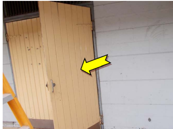
Photo 4. Exterior, throughout, door – suspected lead-containing yellow upper paint system.
