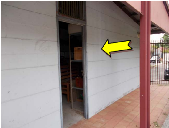
Photo 3. Exterior, throughout, walls and features – suspected lead-containing light blue and red upper coloured paint systems.
